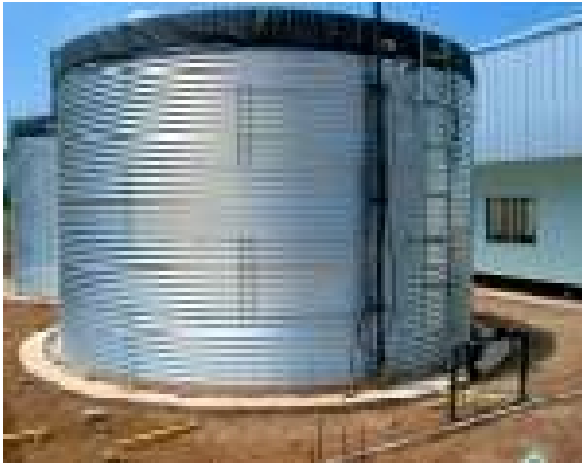
GENAP WATER TANK
